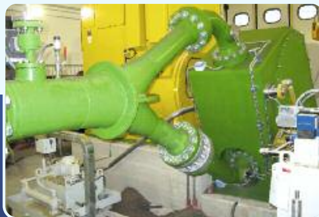
Hydro Power Plant of 1,3 MW in Darzo
